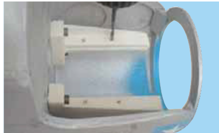
13C- Drill 3/32 in. (2.5mm) pilot holes at right angles through the beams
